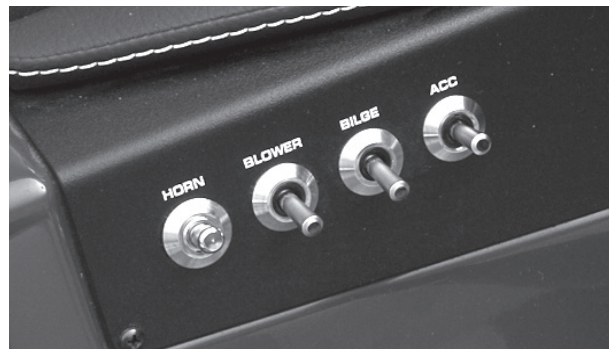
Figure H6: Helm Switch Panel - Port View
