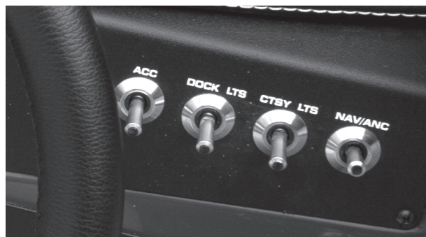
Figure H7: Helm Switch Panel - Starboard View
