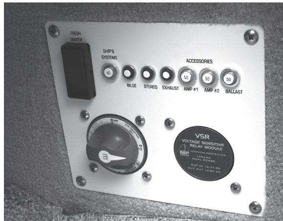
Figure H2: Battery Switch Panel - Stbd Stern Seat Storage (Representative View - Models & Locations May Vary)
