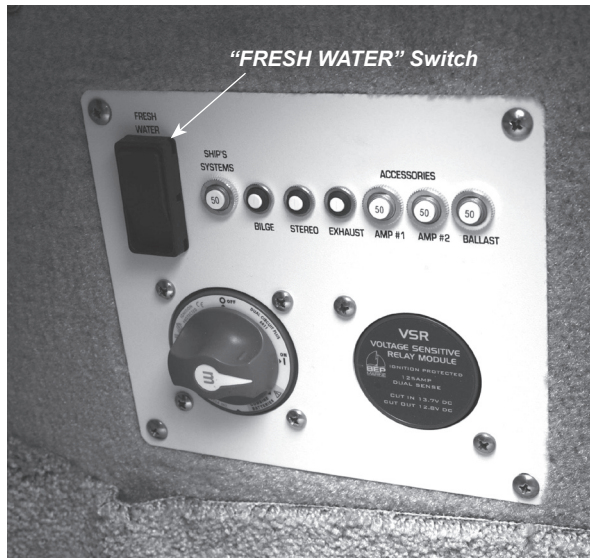
Figure J6: Fresh Water Switch on Battery Switch Panel
