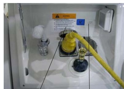
Shore Power Inlet Dockside Inlet Air Warning Label Conditioning Label
