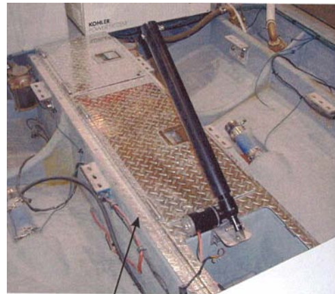
Battery Storage Cover
