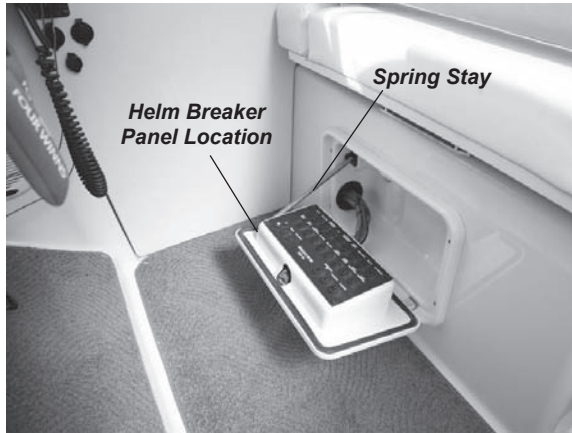
Figure H4: Helm Circuit Breaker Panel Location
