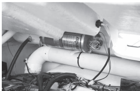
Figure L14: Optional Fire Extinguishing System
