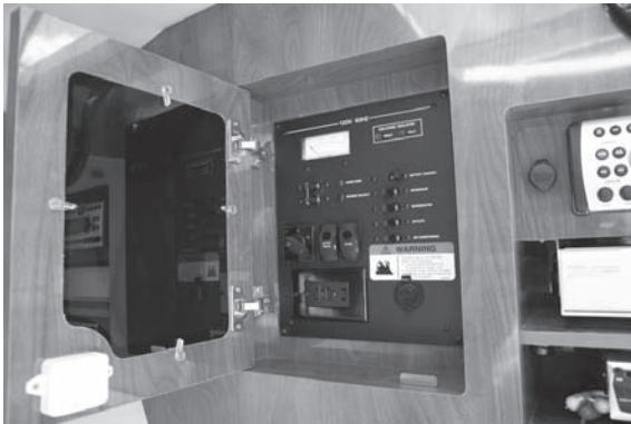
Figure H8: AC Power Panel
