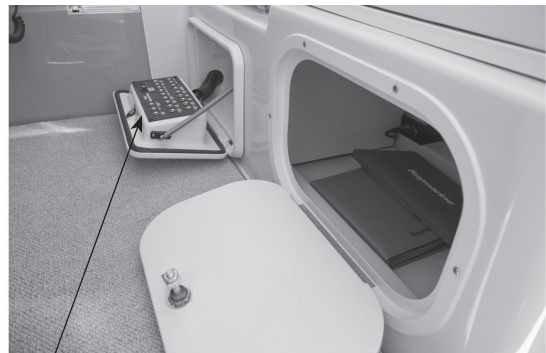
Helm Circuit Breaker Panel
