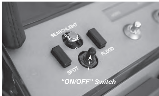
Figure H13: Searchlight Switches
