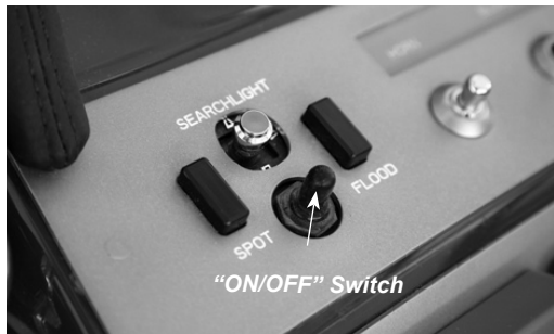
Figure H13: Searchlight Switches
