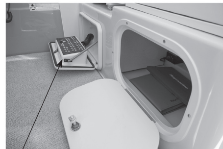
Helm Circuit Breaker Panel
