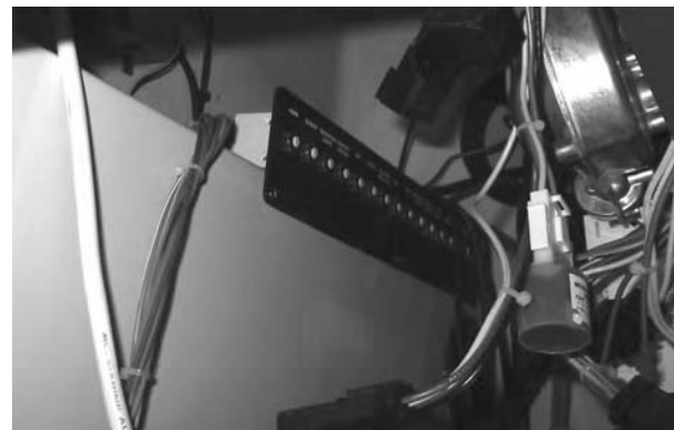
Figure H3: Helm Circuit Breaker Panel Location
