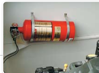
PULL-UP CLEATS FIRE EXTINGUISHER
